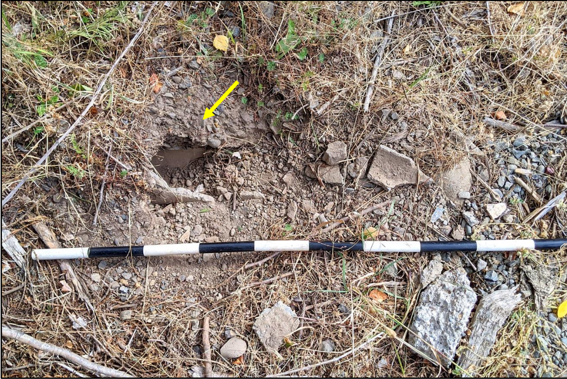
Figure 26. Exposed 6-inch concrete sewer pipe (marked by arrow).
