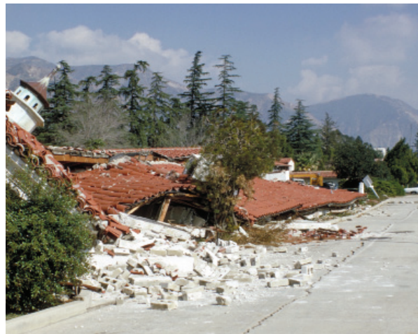
■ Figure 9. Complete collapse of an unreinforced concrete block building, 1971 San Fernando earthquake. —Karl Steinbrugge, NISEE, U.C. Berkeley
