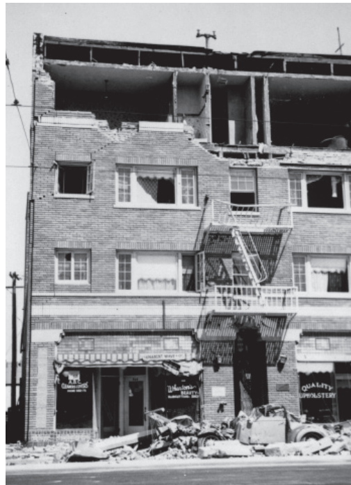
■ Figure 15. URM building damage, 1933 Long Beach, California earthquake. —Los Angeles County Public Library
