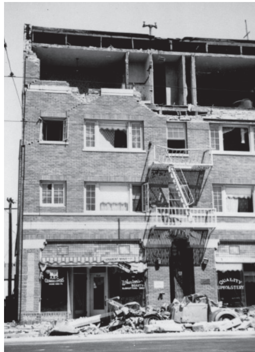
■ Figure 15. URM building damage, 1933 Long Beach, California earthquake. —Los Angeles County Public Library
