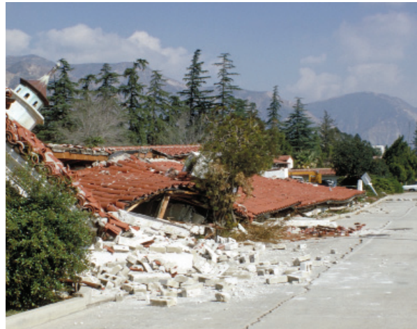
■ Figure 9. Complete collapse of an unreinforced concrete block building, 1971 San Fernando earthquake. —Karl Steinbrugge, NISEE, U.C. Berkeley
