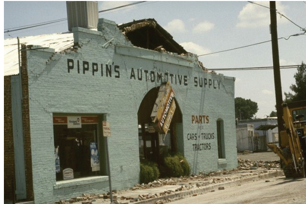
■ Figure 16. URM building with end-wall failure, 1983 Coalinga, California earthquake. Robert Reitherman —NISEE, U.C. Berkeley
