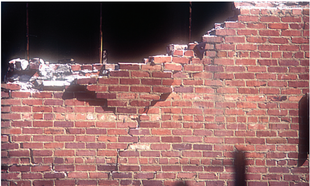
■ Figure 6. Damaged URM wall in a red-tagged building, fated to be torn down or to undergo a multi-year closure for repairs and upgrading.
