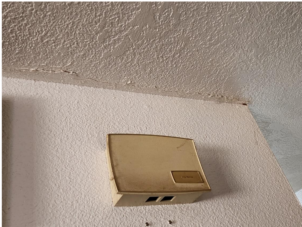
The wall is being lifted and pulling the ceiling sheet rock up, creating a difficult repair.
